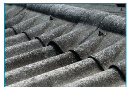
B. Non- Friable Asbestos Example
